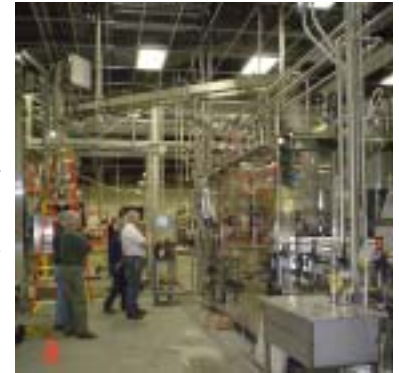
The new bottling line at the Clement Pappas CA facility
