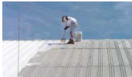
Cranberry grower and part-time Clement Pappas employee, Darren Morris, applies a coating to the receiving station roof.
